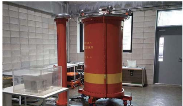
DC 250kV Transformer & Divider
