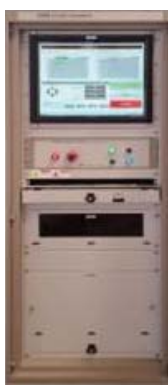
Main PC Control system
